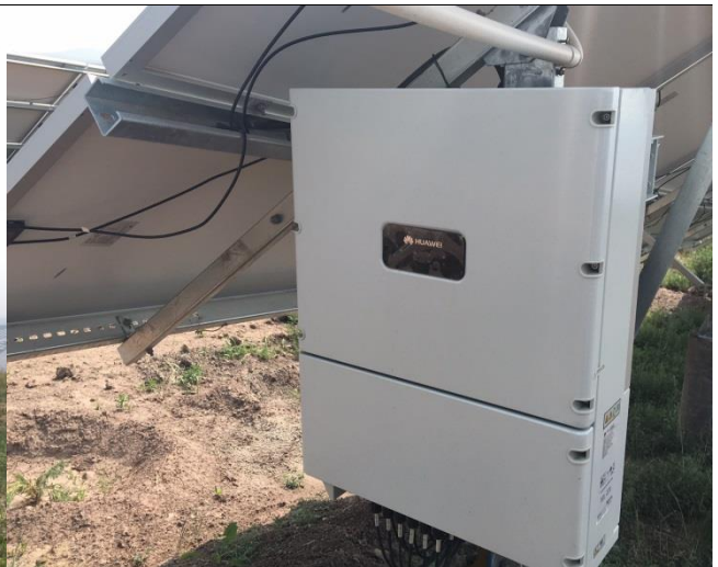
Figure 8: String inverters by Huawei
