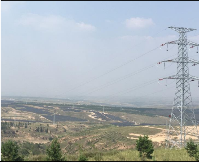
Figure 5: UPV’s Datong project and transmission line
