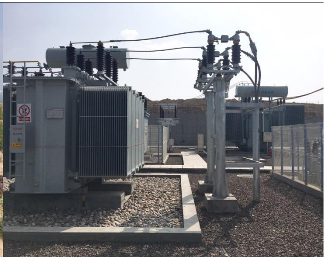
Figure 10: Power transformer for Top Runner base
